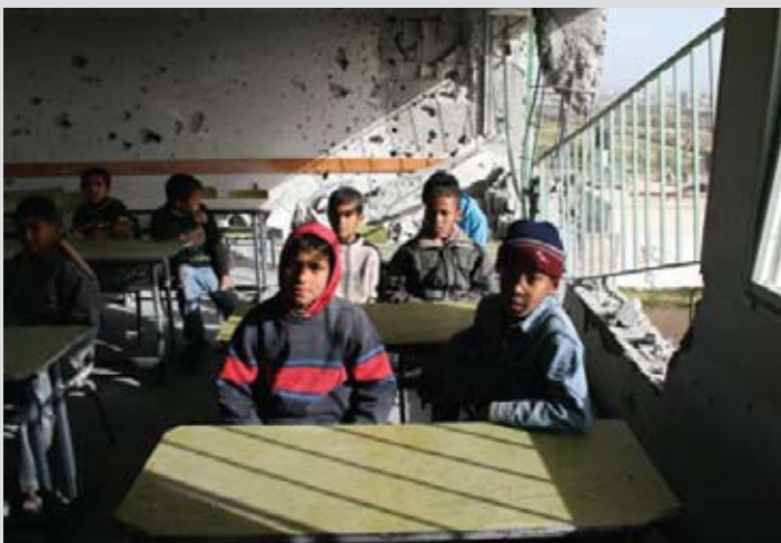
Sixth grade students at the Ghassan Kanafani school in Rafah, South Gaza sit in a partially destroyed classroom. This school is one of the more than 280 schools damaged during the Gaza war in Dec. 2008 - Jan. 2009. PHOTO/Osama Damo
